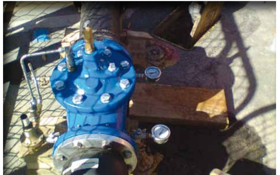
A portable pressure valve which now means large numbers of properties could be kept supplied with water during planned maintenance.
