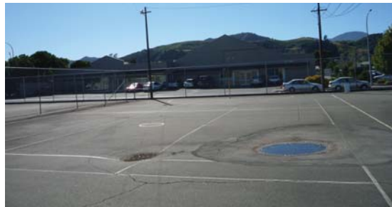
Subsidence is an issue due to unconsolidated fill beneath the surface.
